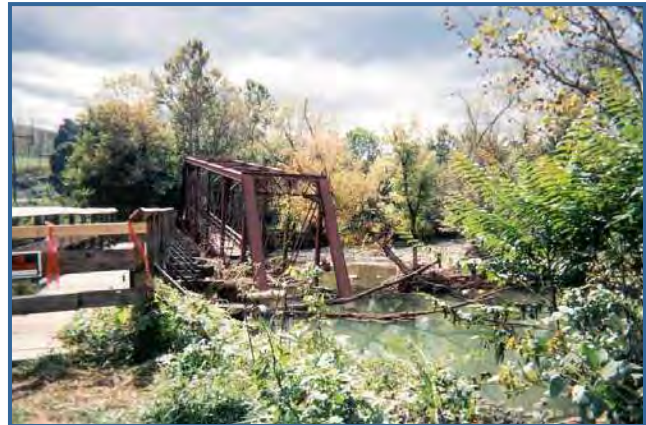
Hurricane Isabel - South River in Rockbridge County
